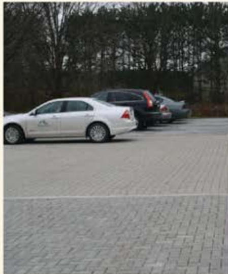
MacMillan is now participating on an American Society of Civil Engineers' committee to develop a standard for permeable concrete pavement.
